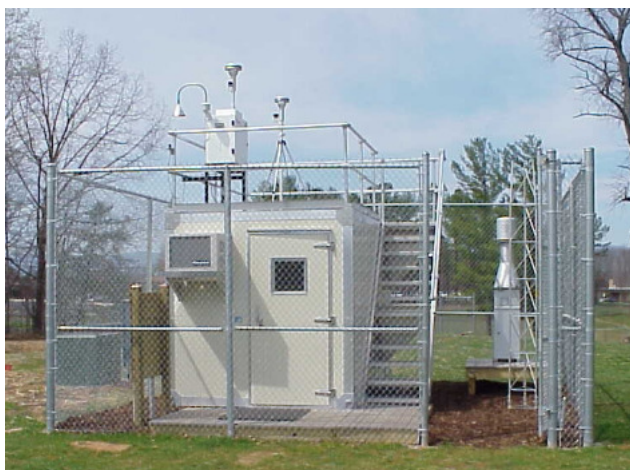
Air Quality Monitoring Station (AQMS)
