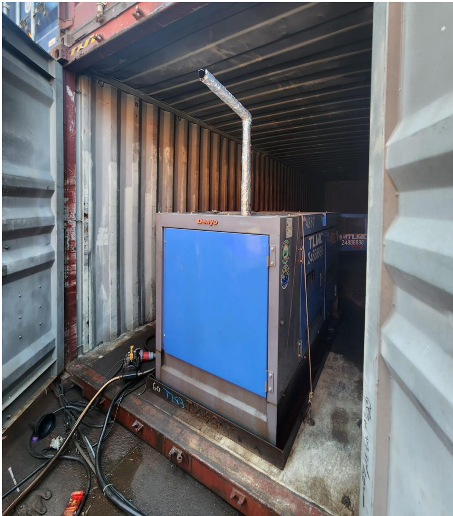
Figure 2: Site Photo of Mobile Generator inside the Cargo Container Taken during the Inspection on 10 January 2025
