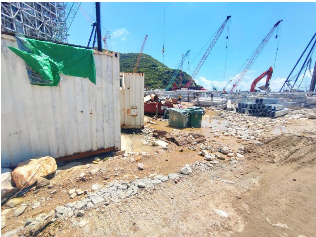
Figure 5: Site Photo of Main Haul Road Taken during Site Inspection on 19 June 2023
