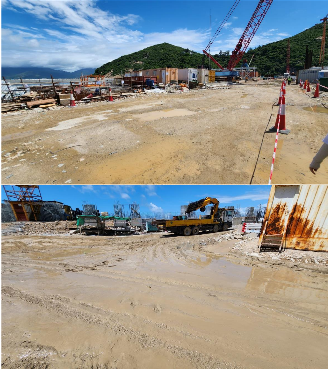
Figure 9: Site Photo of Main Haul Road Taken during Site Inspection on 04 July 2023
