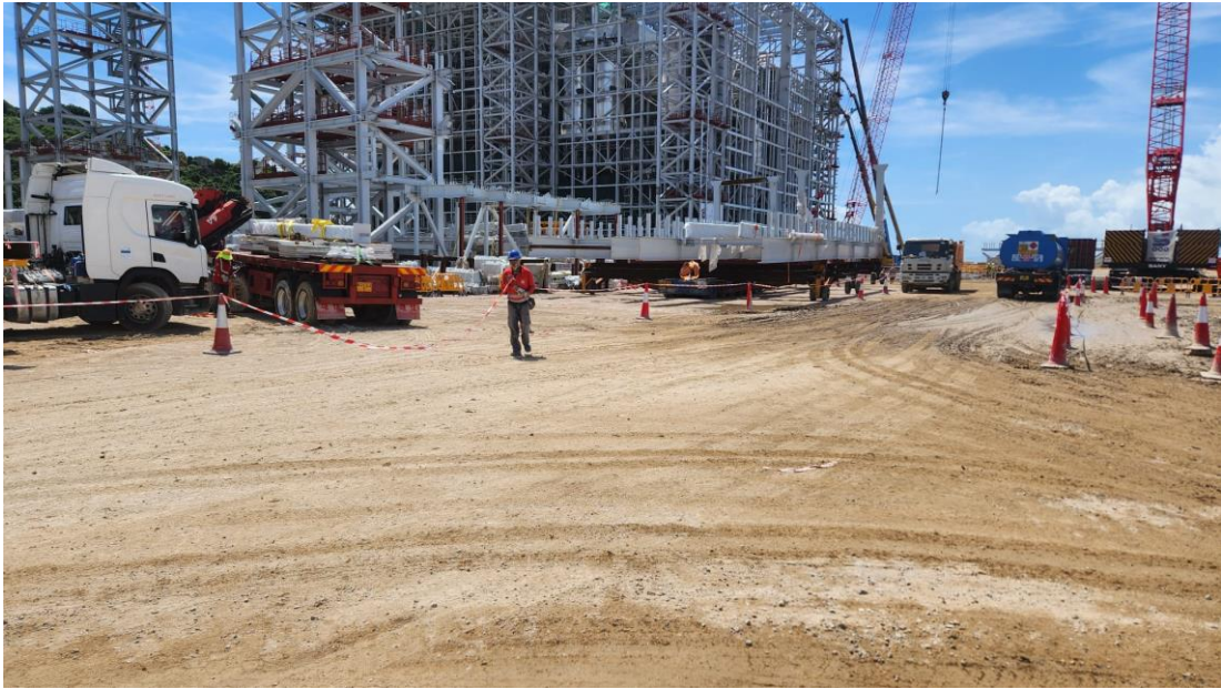
Figure 6: Site Photo of Main Haul Road Taken during Site Inspection on 26 June 2023
