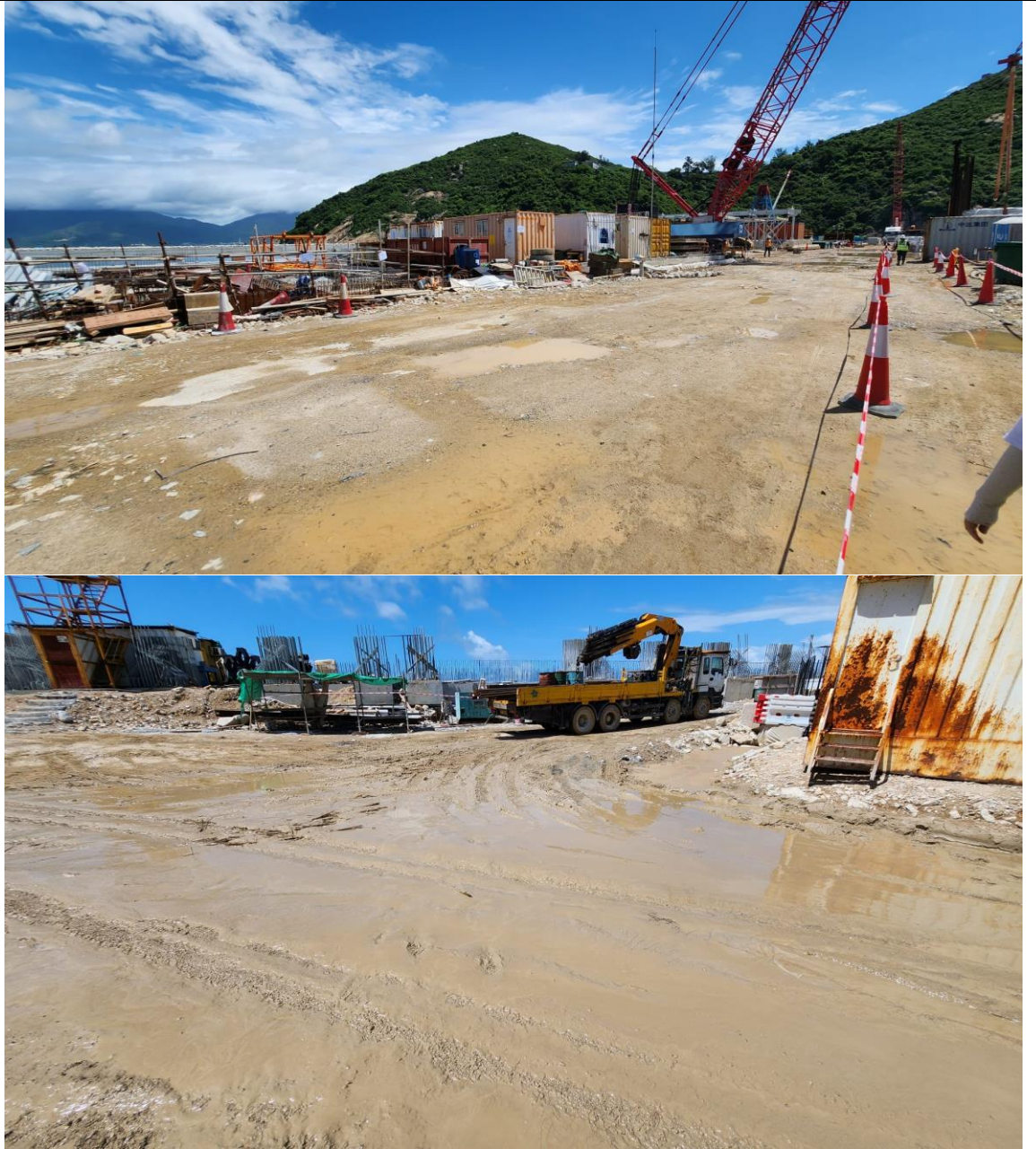
Figure 9: Site Photo of Main Haul Road Taken during Site Inspection on 04 July 2023
